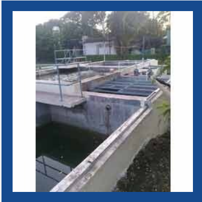
Sewage Treatment Plants
